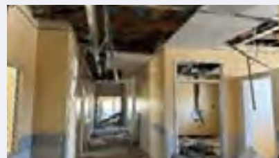
Facility after vandalism
